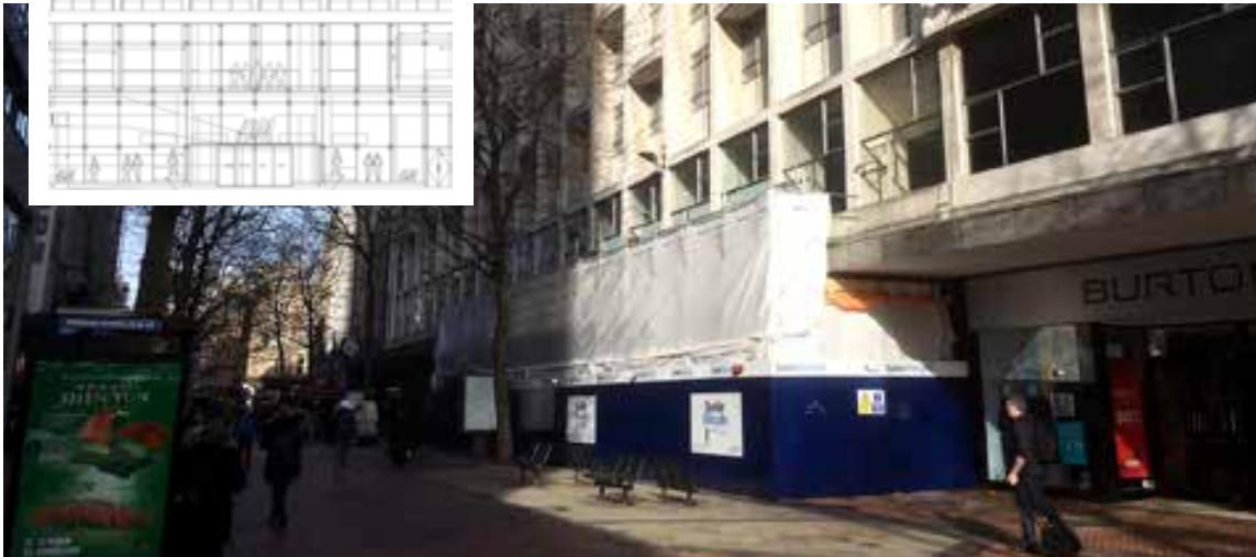
Work underway on the New Street H&M store and one of the planning application visuals for the new frontage, inset
